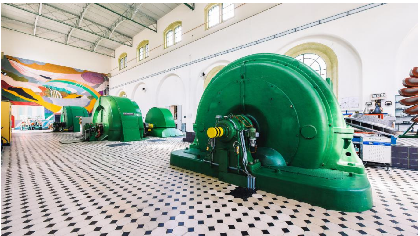
Turbine hall, Robbia power plant
