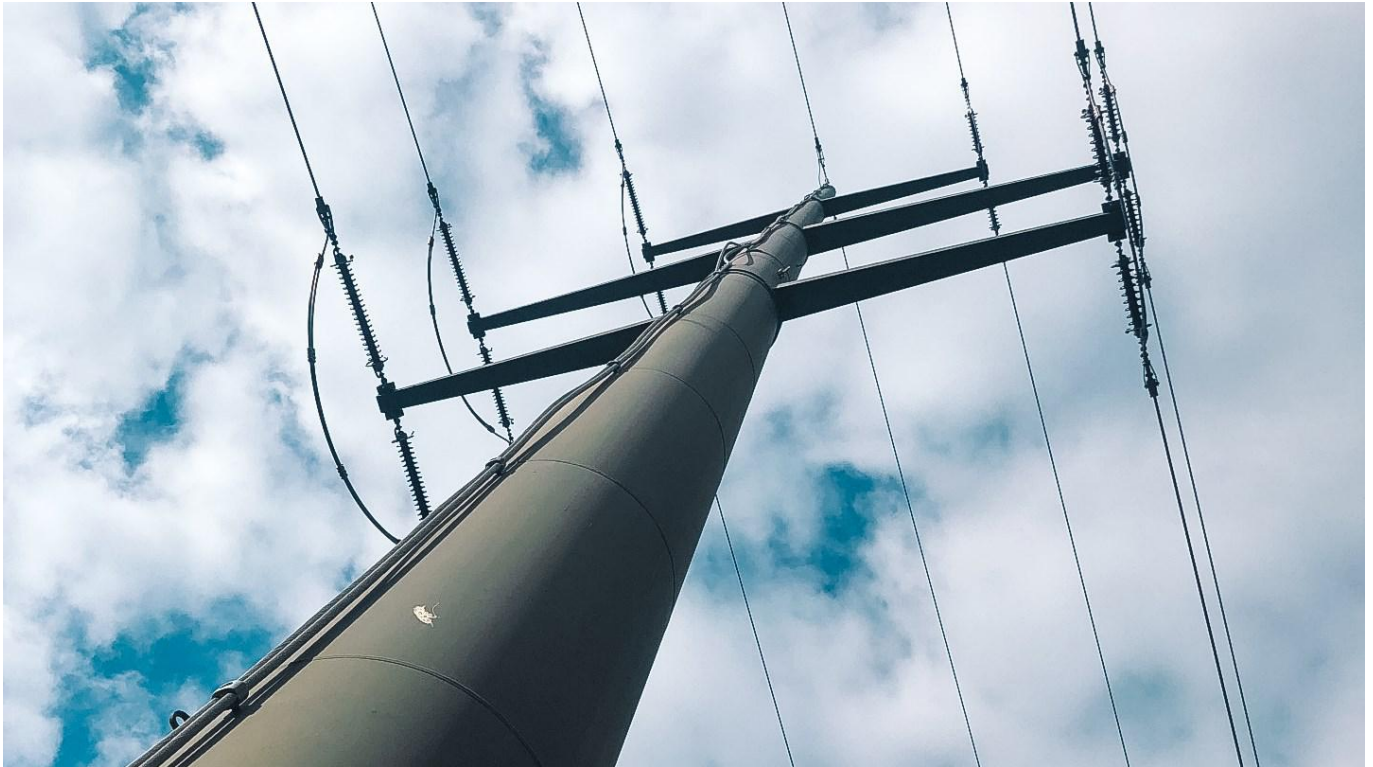
High-voltage twin cable line in the Surselva
