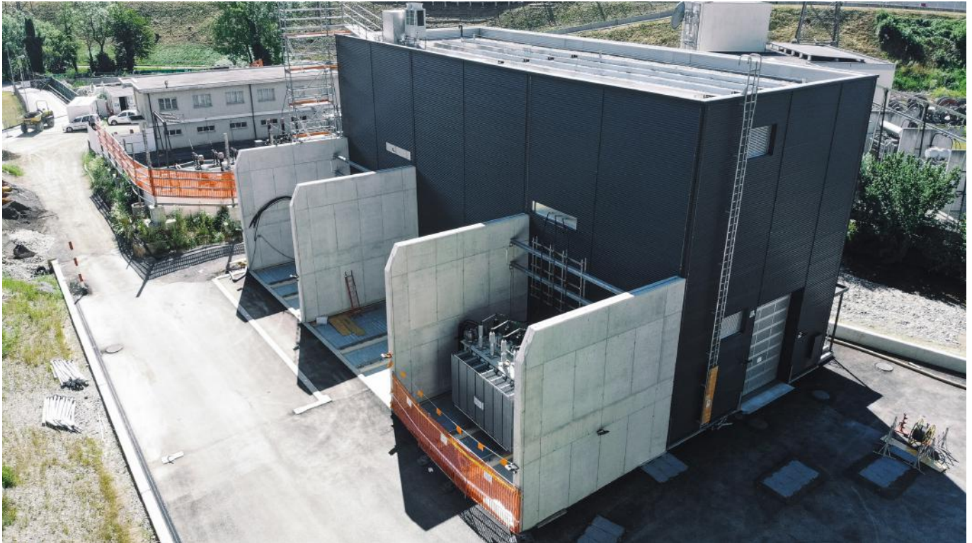
New substation in Mendrisio (Canton Ticino)
